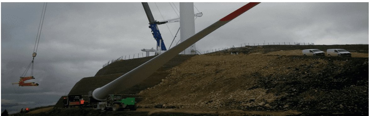
Fig. 7 - installation site of a wind farm
