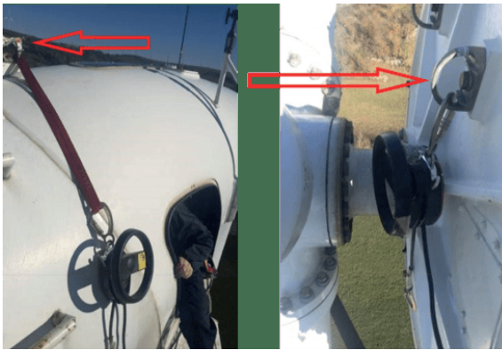
Fig. 6 - small wind turbine
